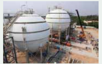
Relocated Spherical Tank
