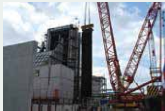
Heat Recovery Steam Generator (HRSG)
